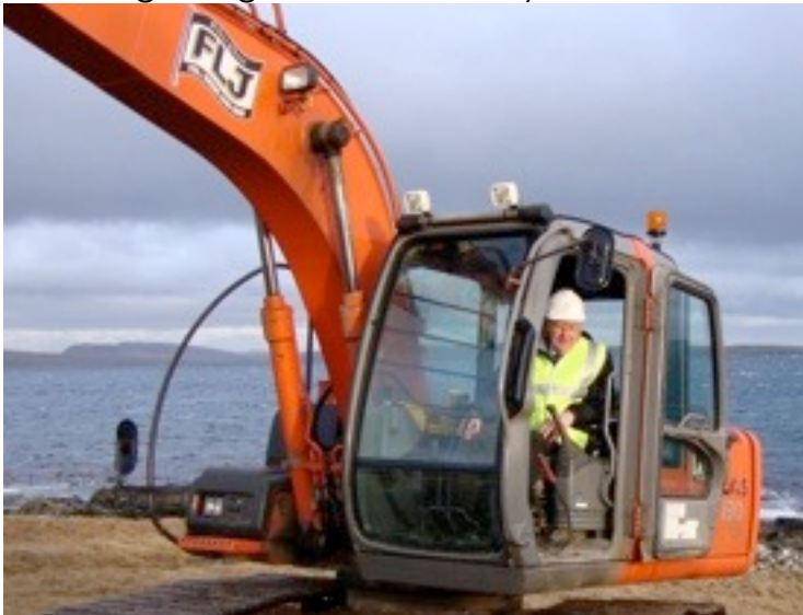
Above- Josie Simpson cuts the first turf at the new breakwater and pier project.
