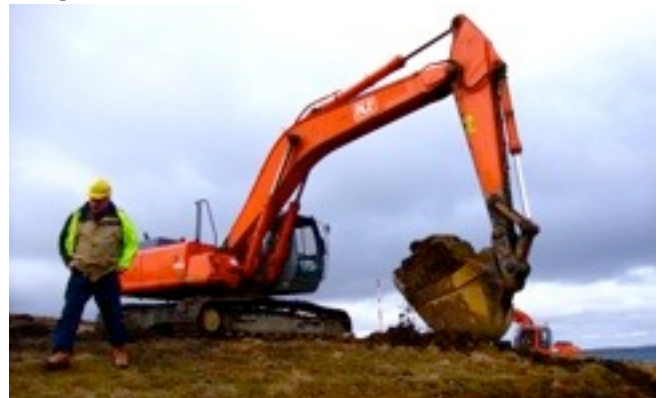
Above - All systems go ! Under direction of contractor Frank Johnson, work on excavating the site begins.
